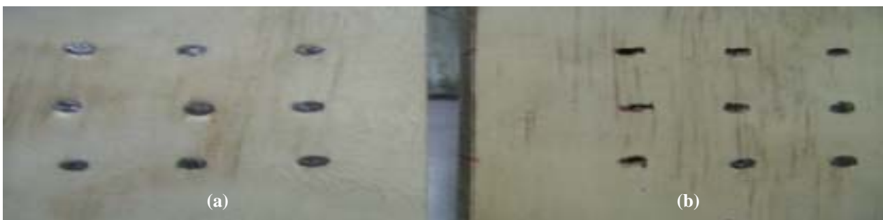
Figure 13. Damage on the outside surface of plywood sides plate, (a) sengon -plywood (b) meranti -plywood
