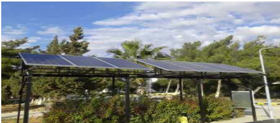
Figure 1 Picture for photovoltaic panel at PFC-DSEER.
