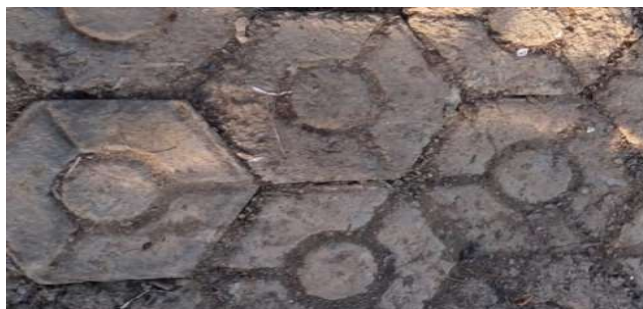
Figure 2 Plastic paving blocks on day 365.
