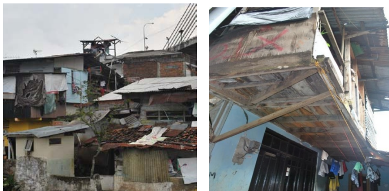
Figure 5. Vertical 'set-above' housing changes reflecting multiple housing form types and building methods
