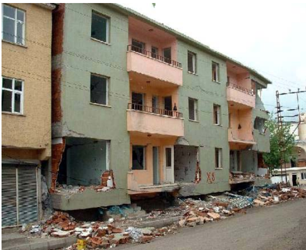
Gambar 1. Soft-storey - Gempa Bingol, Turki 2003
