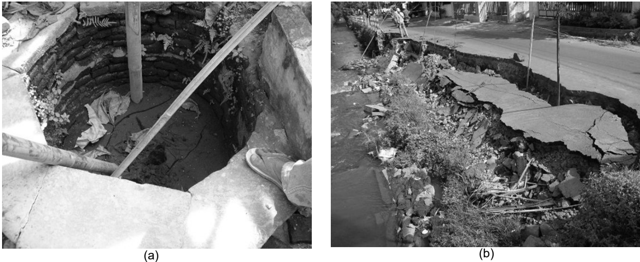
Figure 1. Liquefaction phenomena found in Yogyakarta 2006 (a) sand boiling in an open well (Adi, 2013) (b) lateral spreading on edge state road (Adi, 2013)
