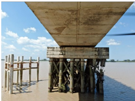
Figure 2. Damage in pedamaran II bridge foundation
