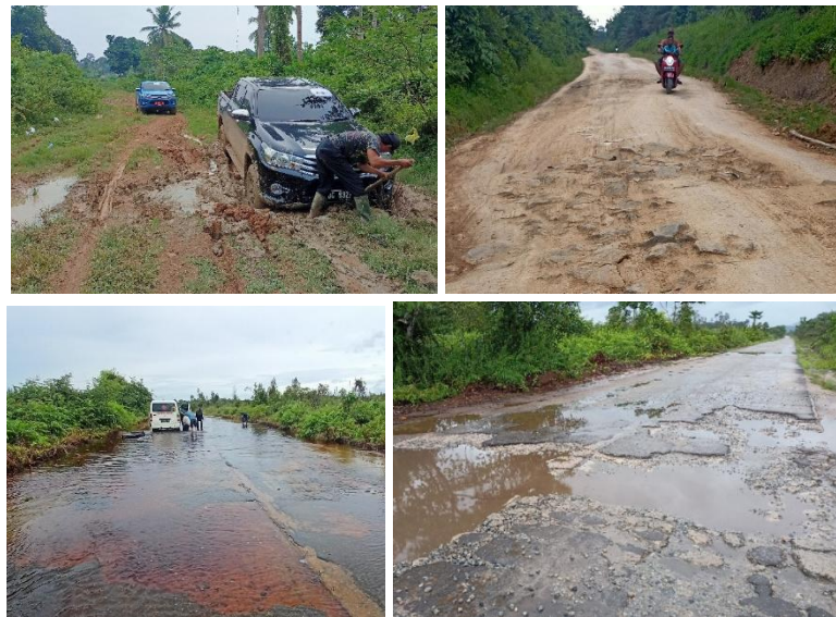
Figure 1. Examples of road failure based on investigation findings conducted across Indonesia
